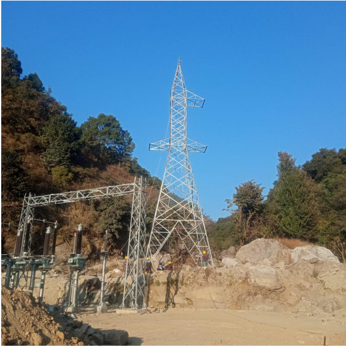
Figure: API Tower at Powerhouse Switchyards
