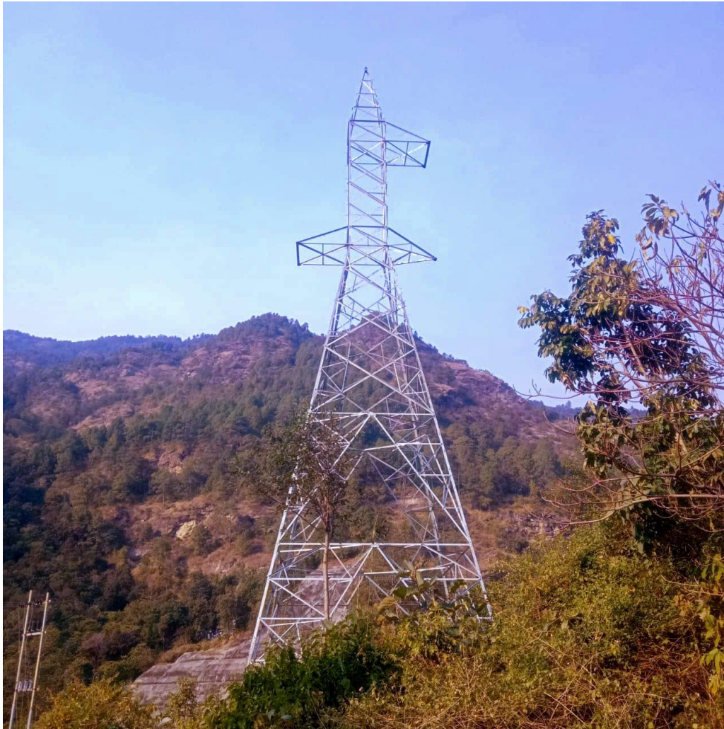
AP2 Tower at Powerhouse Switchyards
